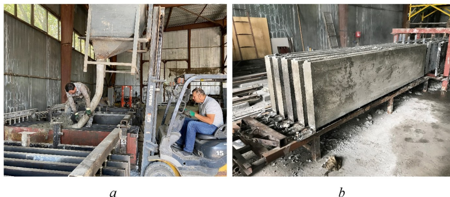
Figure 3 - Forming panels on a cassette installation (a) and unmolded panels (b) DOI: https://doi.org/10.60797/mca.2024.55.1.6
